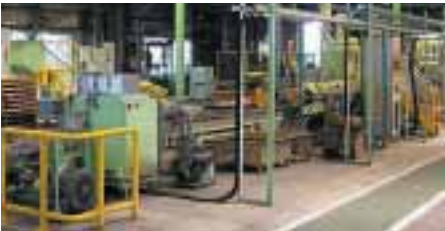
Pelletizing equipment at the Kuwana Works
