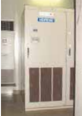
Inverter power source equipment
