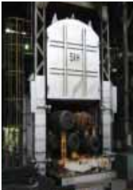
Heat treating furnace
