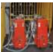
Cast-frame hydraulic cylinders were changed to electric-powered servo cylinders
