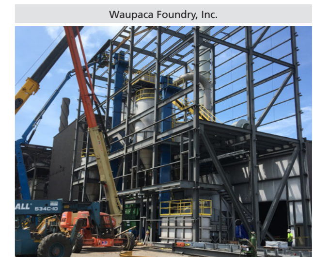
Sand recycling system adopted by Plant 5
